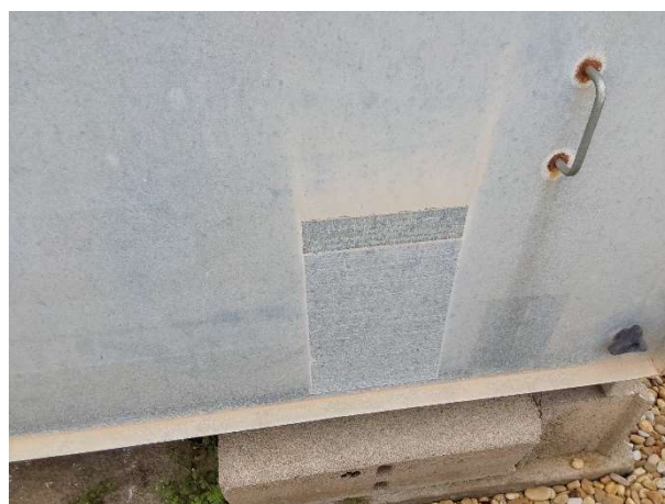
Plaque signalétique illisible
